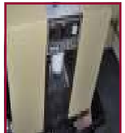
Equipment in Place
