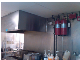
5' Long Fire Suppression System (2) PCL – 300 Extinguishers
