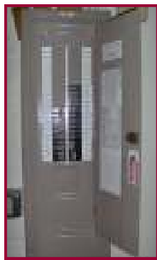
200 Amp Electric Service Panel
